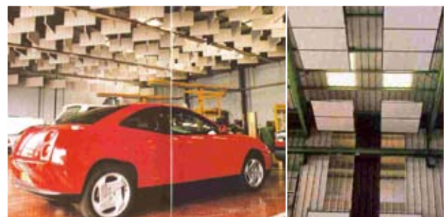
Figure 4.19 Garage – Room absorption (© Yves Cousson – Courtesy of INRS – France)
